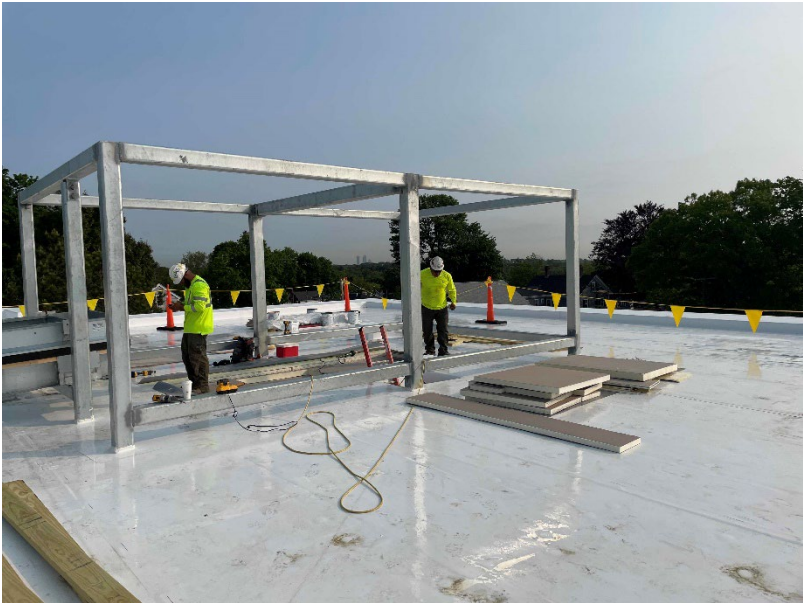
Mechanical Structure on roof
